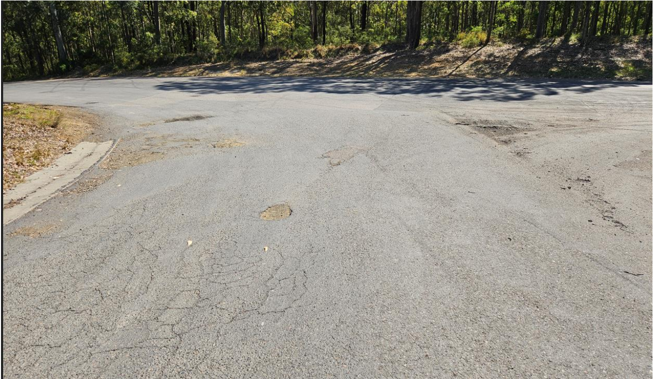
Plate 3.3 Pavement cracks on Quarry Access Road at Black Hill Road intersection
